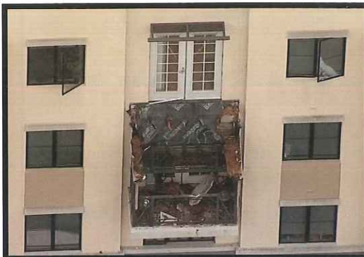
Berkeley Balcony Failure (CBS)
