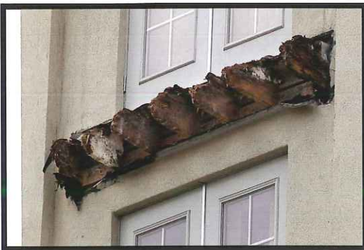
Damage found to structure following the Berkeley collapse in June 2015. Image: Jeff Chiu/Associated Press
